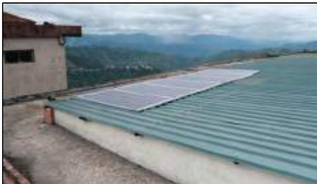
Rooftop Solar Panel
