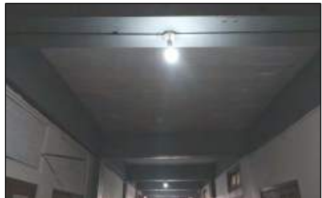
Hallway LED light
