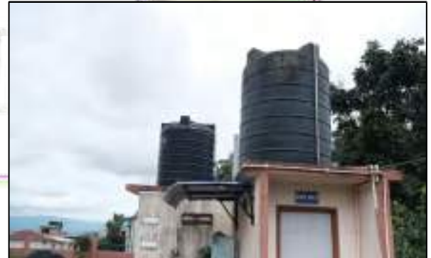
Rooftop Water Storage Tank
